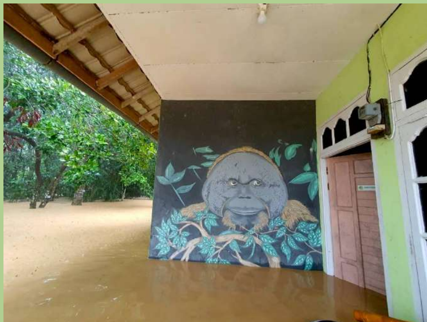
Floods submerged Bentangor Environmental Education Center in Pampang Harapan Village. The building sits atop wooden stilts. Pictured here is the elevated front porch of the building. The dirt road and wooden floorboards have been covered by water.
